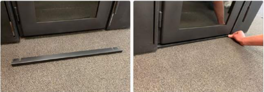
Insert the bottom trim piece under the stove, so it rests on the masonry and is flush with the other trim pieces.
